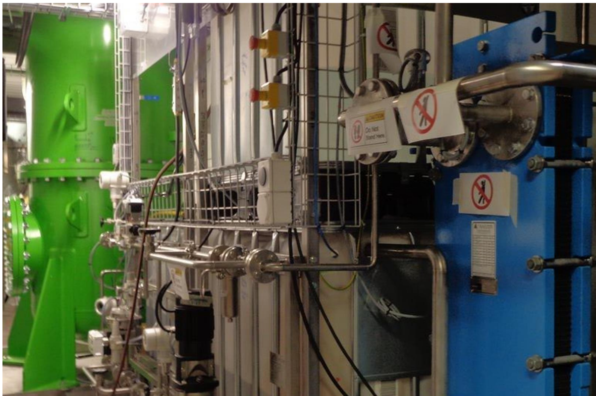
Figure 6. SulPure® Main Process Line container
