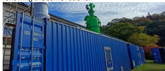
Figure 2. SulPure ® prototype installed at the Maritime Centre of Flensburg University of Applied Sciences (Hochschule Flensburg).
